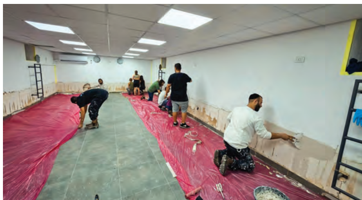
Renovating a bomb shelter which was flooded by 50 cm of water and sewage. This shelter is designed to shelter some 30 families during missile attacks.
