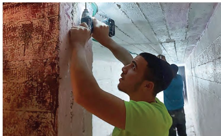
Tenufa Bakehila work team making urgent repairs to bomb shelters in Israel’s north.
